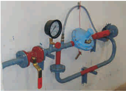
Commercial Gas Pipelines
