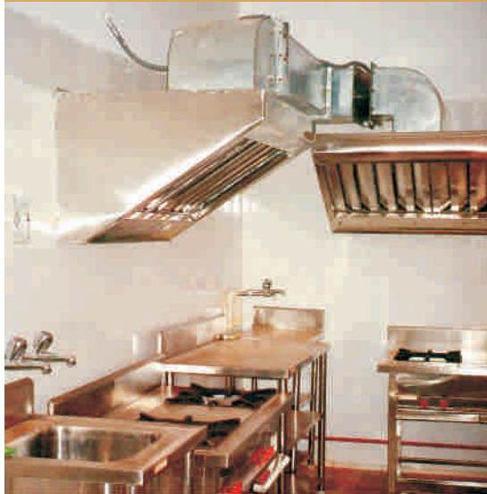
Hood with Ducting
